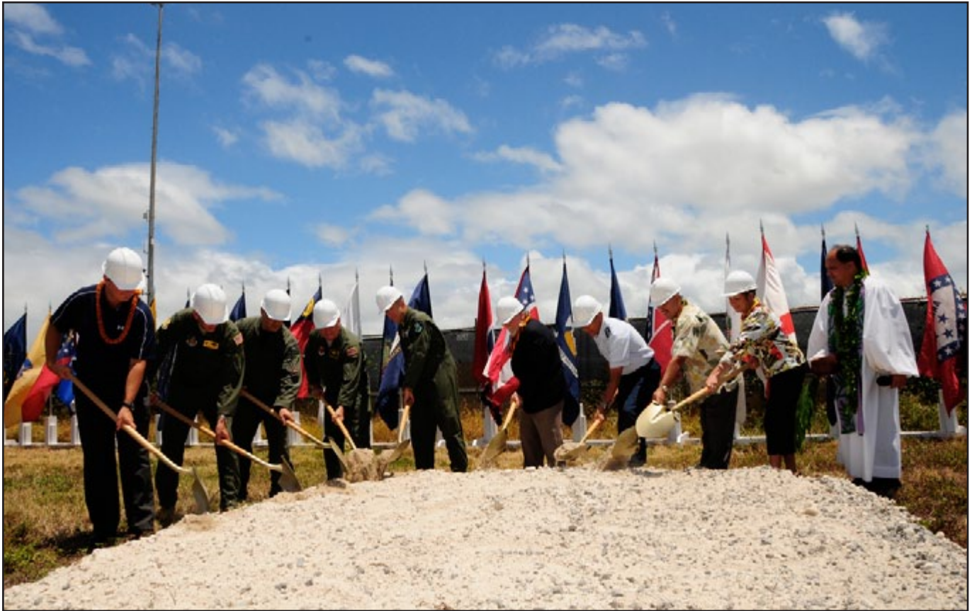
Dignitaries invited to ceremoniously “break ground” turn the dirt on the Hawaii Air National Guard’s new state-of-the-art F22 maintenance facility July 22, 2011 at Joint Base Pearl Harbor Hickam. Governor Neil Abercrombie, and The State Adjutant General Darryll D.M. Wong presided over the ceremony.
